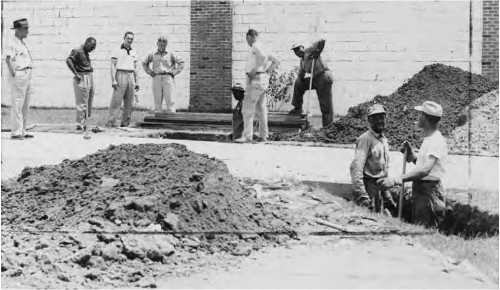
FIGURE 7. African American workers, possibly incarcerated persons from the Sandy Point correctional camp, unearth the damaged sewage pipe that was used as an excuse to close the park following Judge Chesnut's injunction in June 1953. Courtesy of the Afro-American Newspapers Archives
